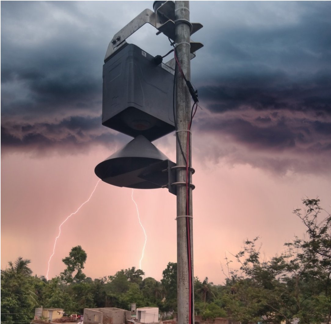
Earth Networks Sferic Siren installation in Odisha
